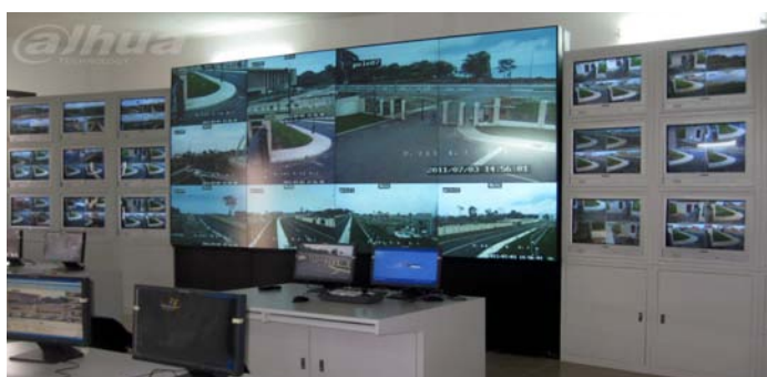
National Grid project in Equatorial Guinea Video Wall 3x4
