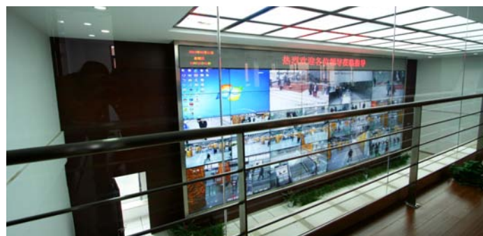
Hangzhou Subway Public Security Bureau Video Wall 6x8
