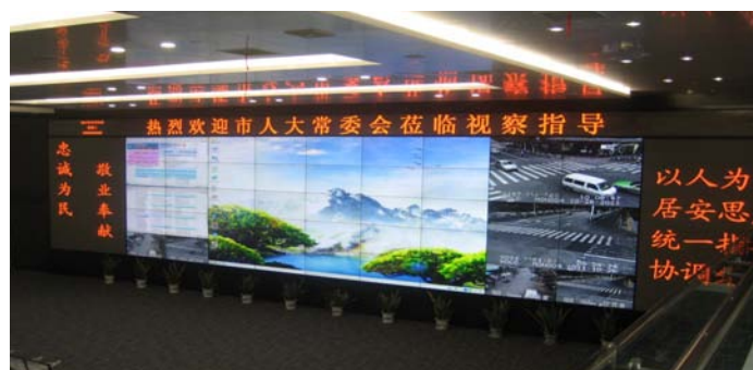
Public Security Bureau in Jiangsu Province Video Wall 5x9
