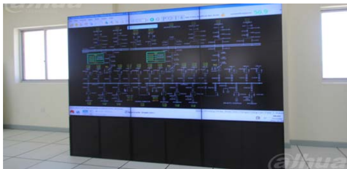
National Grid Project in Dili, East Timor Video Wall 3x3
